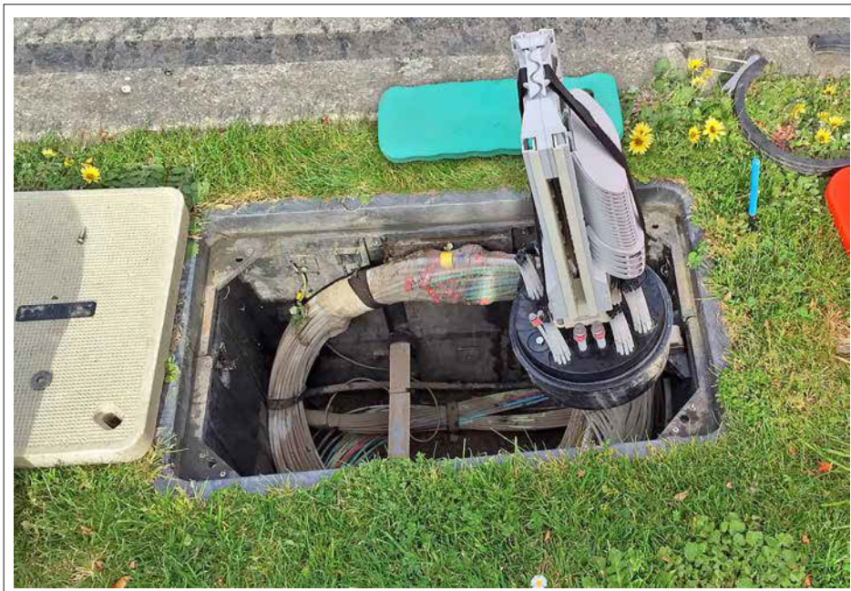
Figure 4 Example of a typical fibre access point, Lower Hutt
